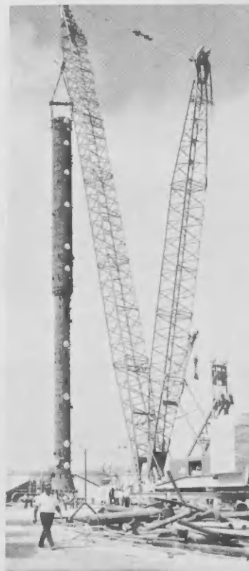
Fingering the sky here are the V-shaped boom and mast of the Manitowoc Crane setting one of the catacarb towers in place.
